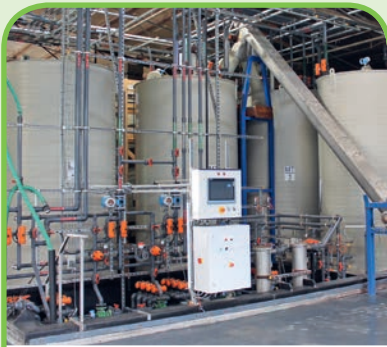
New mixing equipment
